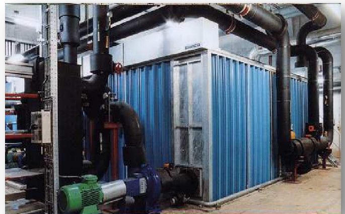
An hybrid tank, installed indoor on a pharmaceutical site. On the bottom we can see the outlet flange for water loop.
