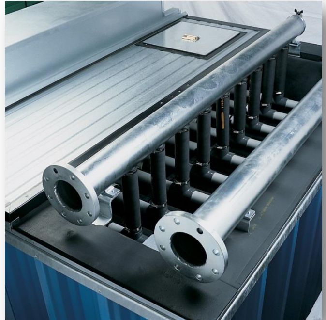
Main headers for water loop and glycol loop (inlets)
