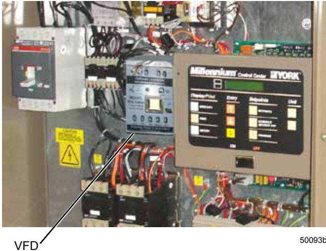
FIGURE 45 - TYPICAL VFD LOCATION
